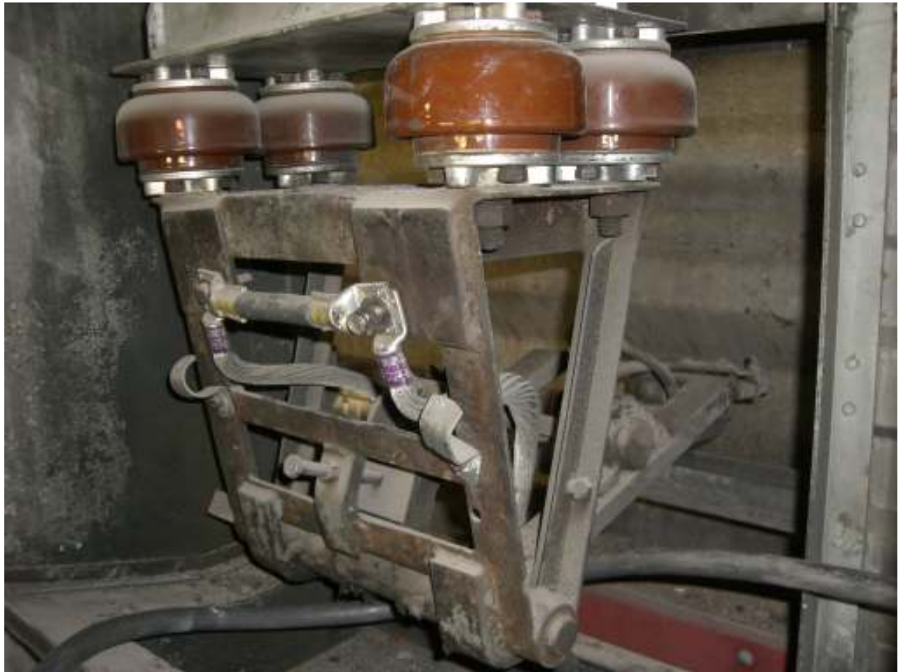
Negative Collector Assembly installed in collector compartment
